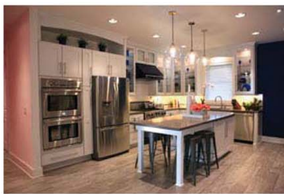
Installed LED recessed lighting from Lighting Science Group
